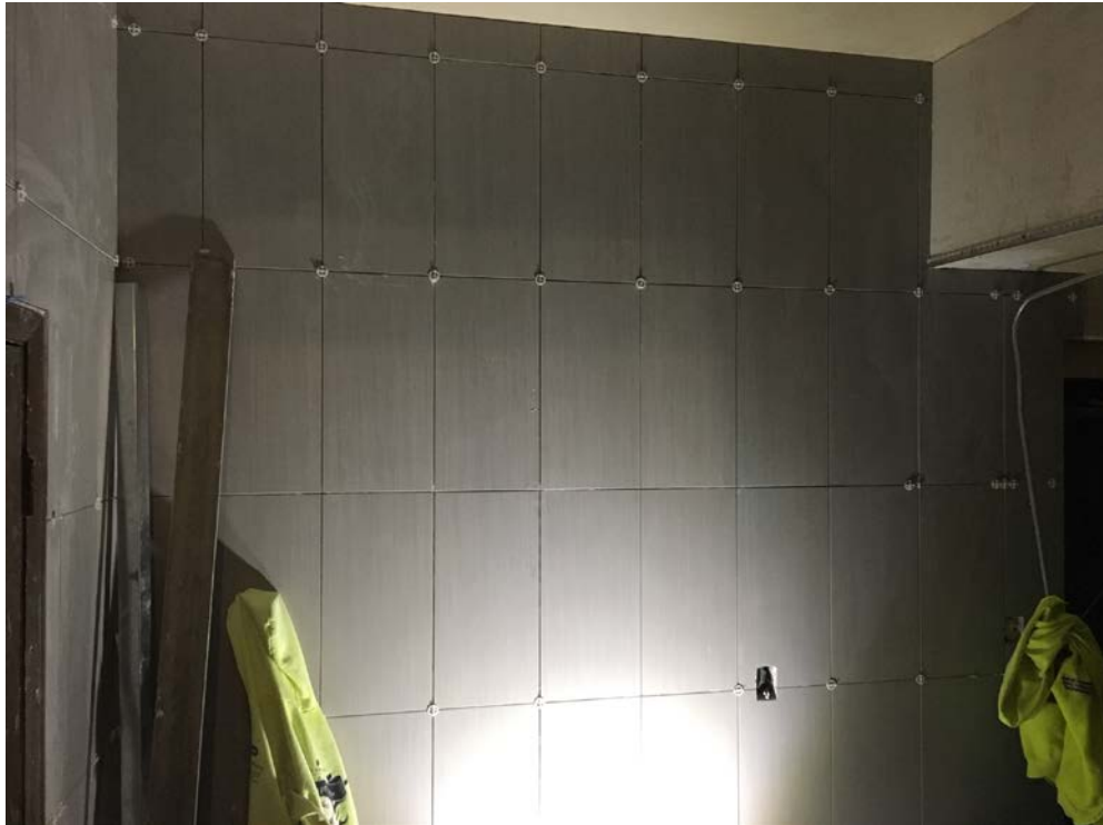
Ceramic tile work at the exit stairway leading out from the HS Locker Rooms.
