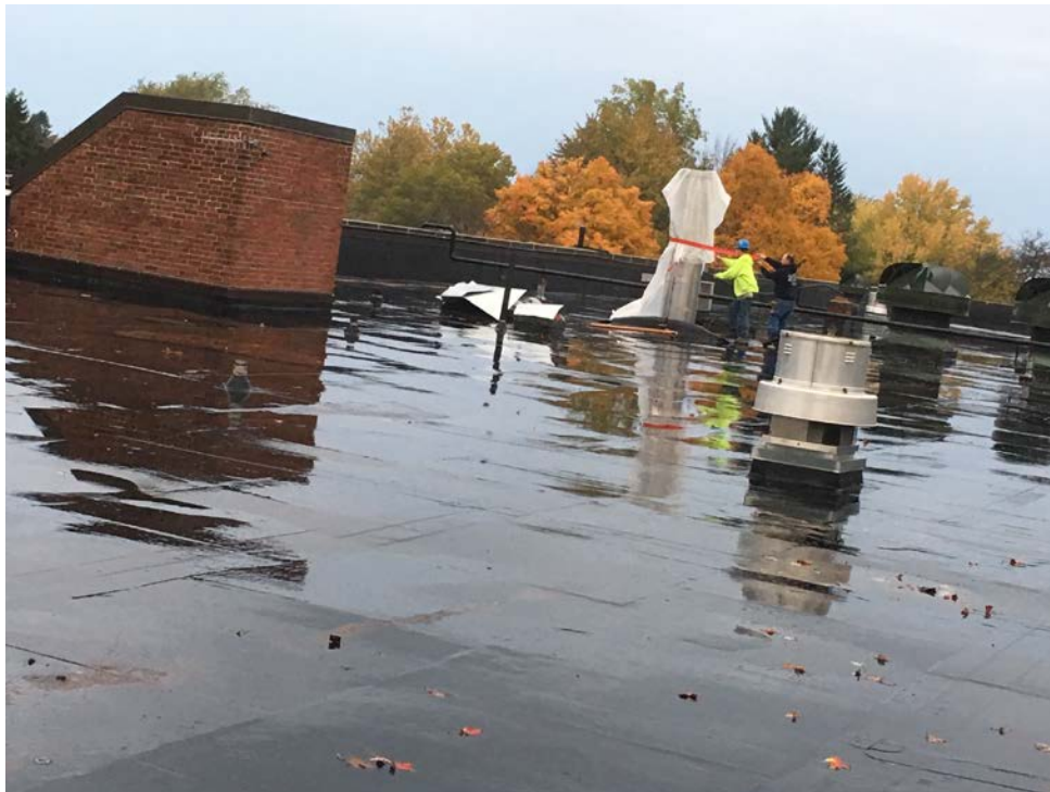
October's nearly continuous rains, made cause for further temporary protection to be needed on the roof of the Middle School.
